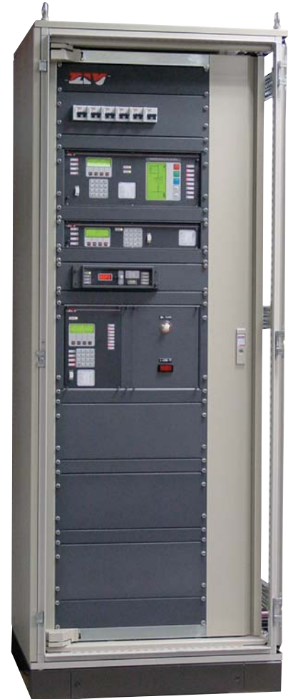
Protection and control cabinet
